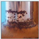
Corrosion on hydraulic rod
